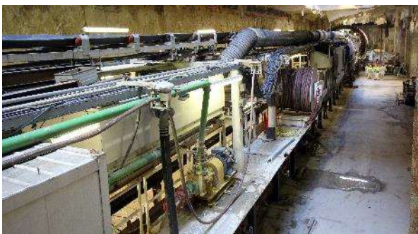
Back up TBM
